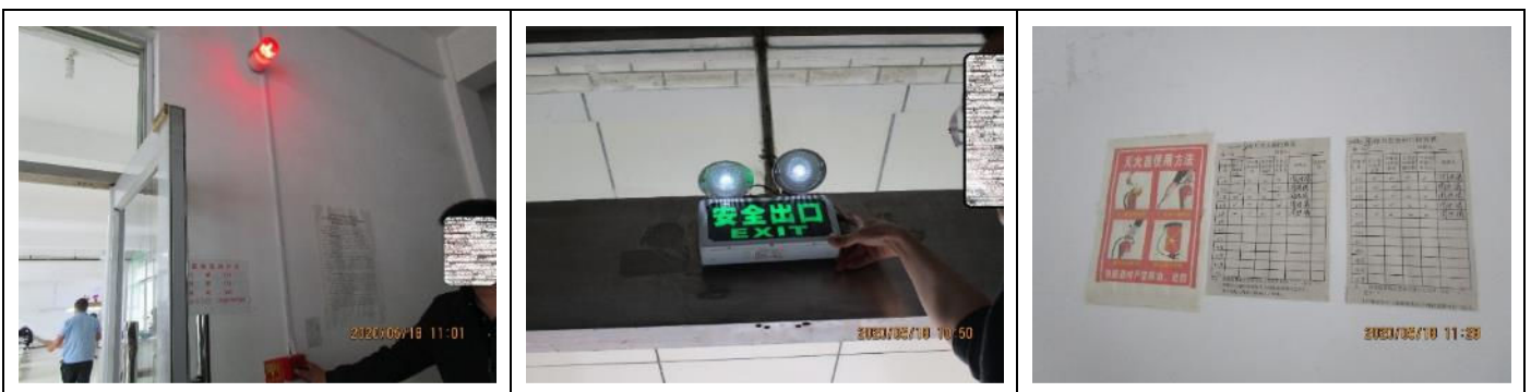
Testing fire alarm Testing emergency light Fire-fighting equipment inspection record
